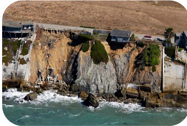
Failing seawalls at Gleason’s Beach, Sonoma County, 2005
